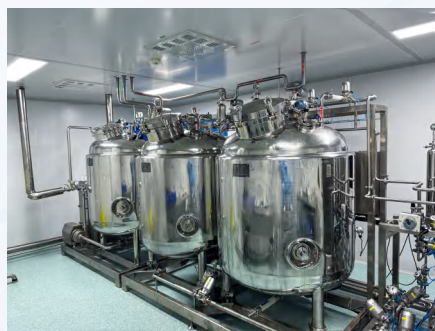
CIP/SIP Compounding System
