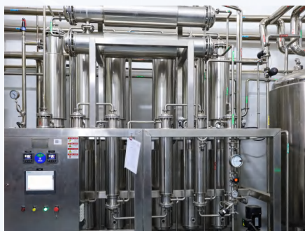
WFI Generation System
